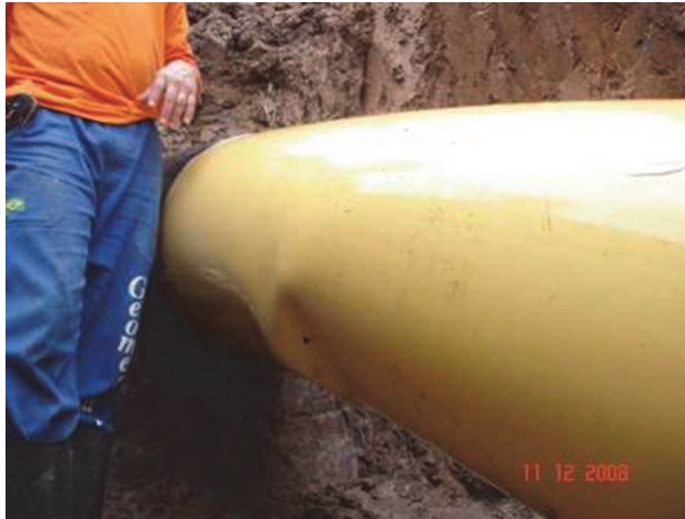
Figure 1.2 Pipeline with local buckling created by soil movement (figure courtesy of Pacheco et al. 5 ).
