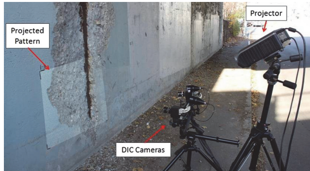
Figure 8.15 Experimental setup for projected pattern measurement to quantify spalling on a bridge in Lowell, MA (reprinted from Nonis et al. 46 with permission).
