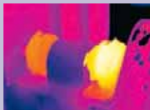
Overheating bearing cap
