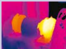
Overheating bearing cap
