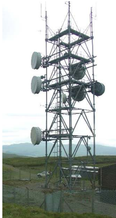
Figure 6a. Microwave repeater showing multiple co-located antennas. 3
