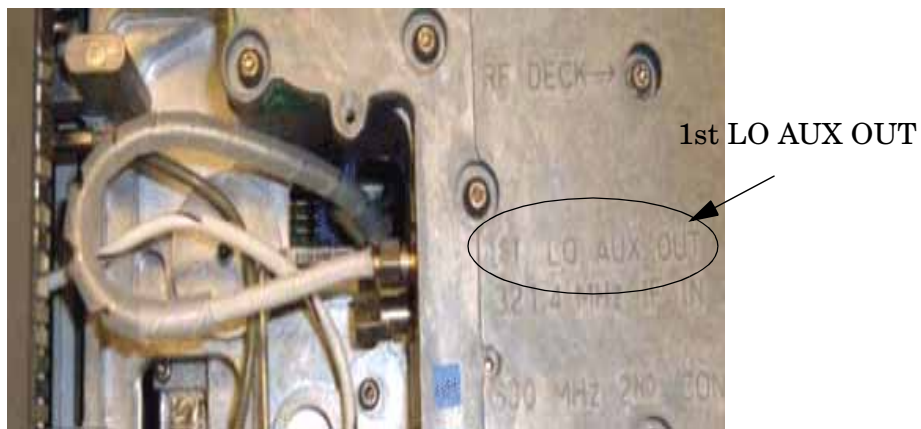
Figure 5 Spiral Wrapped Cable to 1st LO AUX OUT
