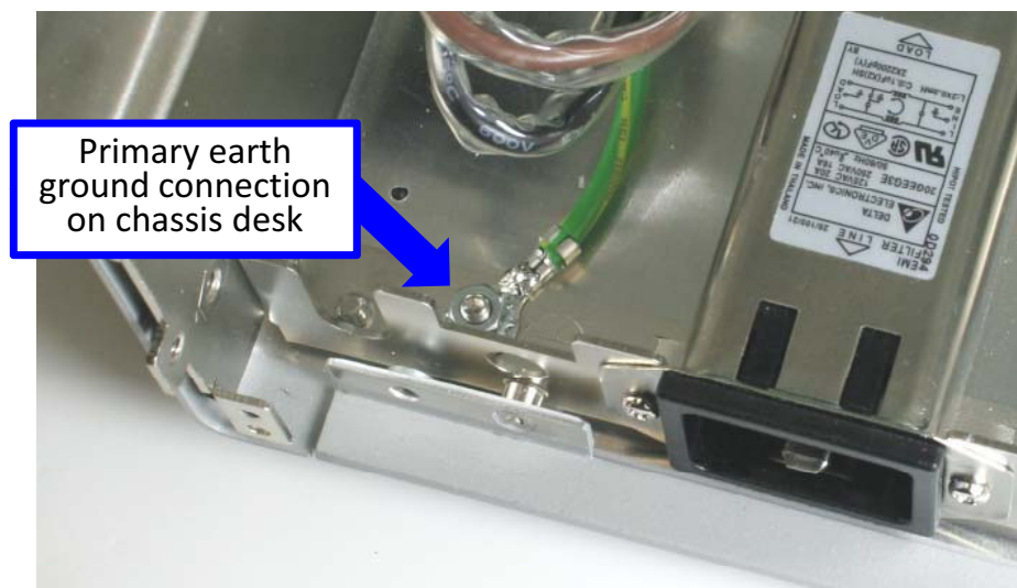
Figure 96 Measure the resistance from the power supply enclosure to the primary earth ground connection on the chassis deck.
