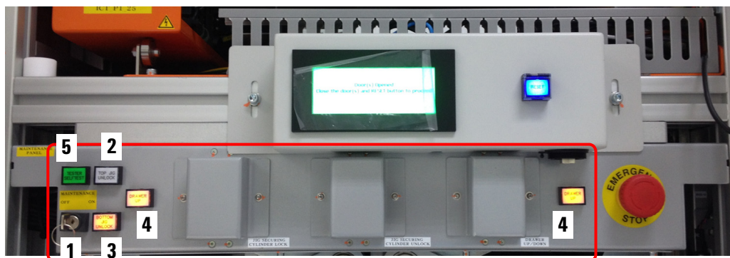
Figure 1-5 Manual Control Panel
