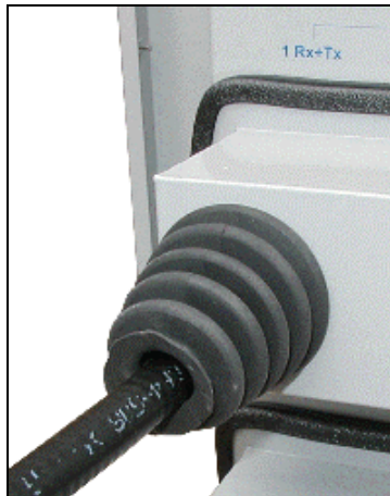
Figure 16. Cable, Connector Boot, and Cover Attached to the Cabinet
