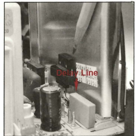
Fig. 11: The large square object is the comb filter delay line. Inject VA62 substitute signals at the output and the input of the comb filter to determine if it's the cause of poor video.
