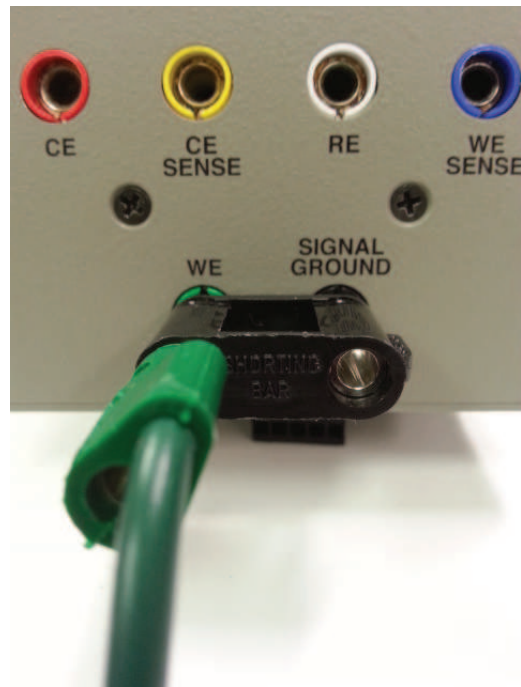
Figure 15: Grounding WE at the EC19.
