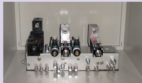
Hydraulic valves mounted in separate cabinet by the machine
