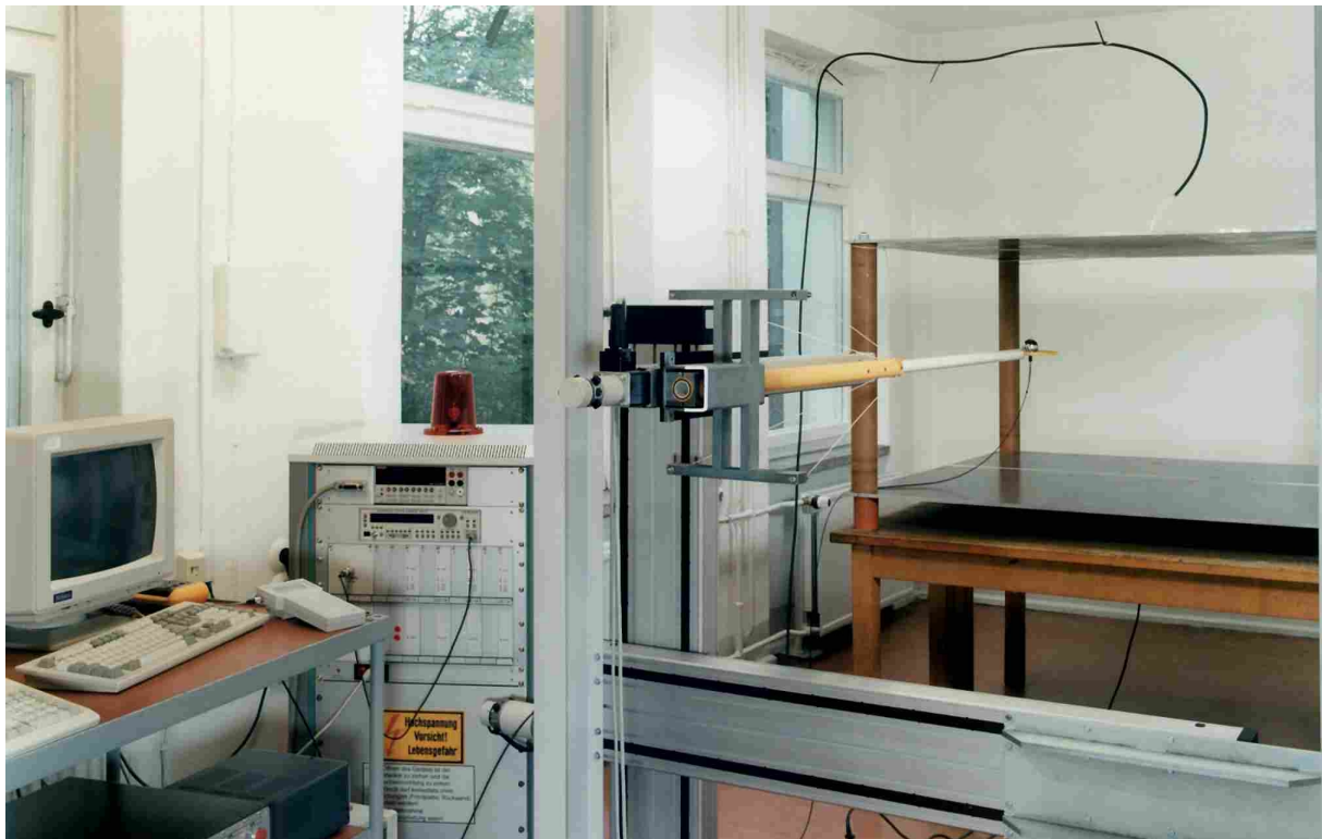
Figure 4: Field generating and measuring device - computer-controlled HV generator in a movable rack (under the window) - three stable axes of the positioning system in the foreground - low dielectric carrier with the probe on its end, moved by the different axes - plate system held by special low-dielectric tubes
