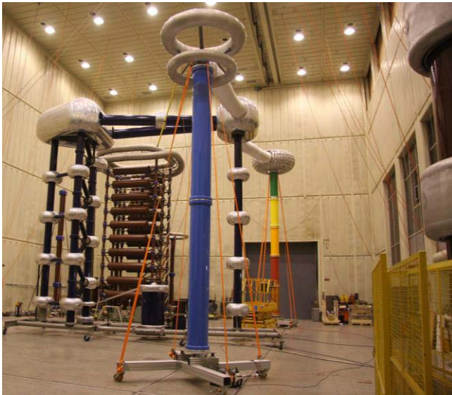
Fig. 8. Setup with the reference divider (in front), the generator with divider (in the middle), and the modular divider (in the background) [9], during the intercomparison at Aalto University's high-voltage laboratory.
