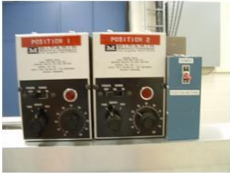
Chamber alignment controls 300 kV range
